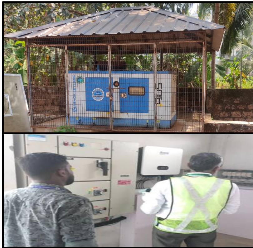
Energy conservation facilities observed in the Campus
